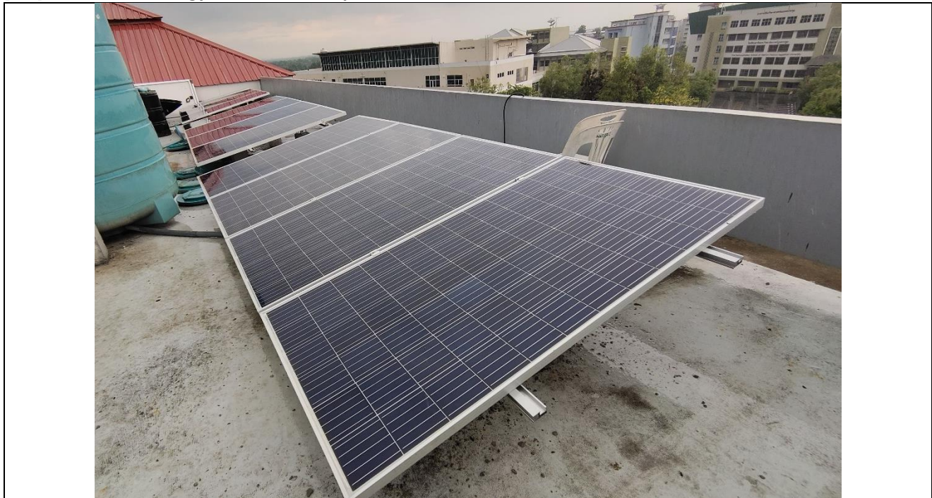
Example of 3.96 kW Solar Roof Top (Engineering and Technology Building)
