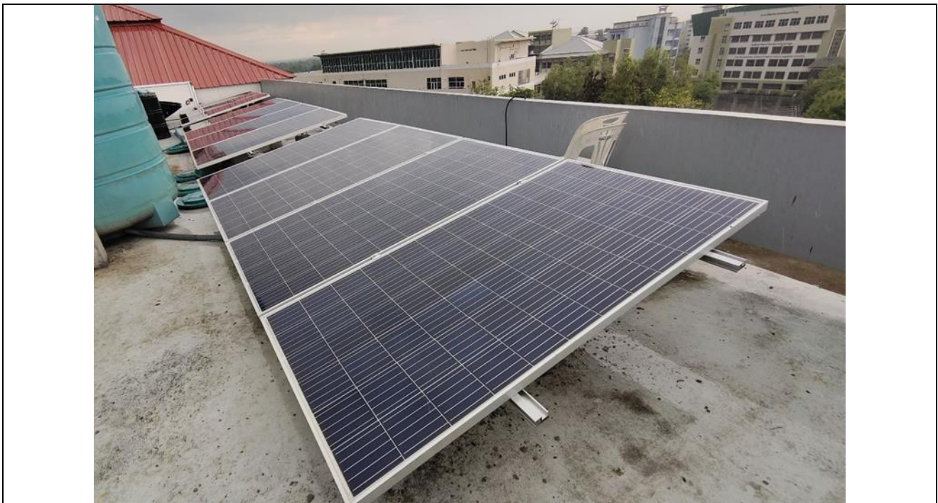
Example of 3.96 kW Solar Roof Top (Engineering and Technology Building).
