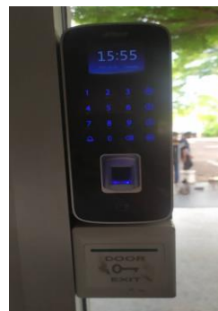
[S1]-Intruder alarm of Siri Varapunya building.
