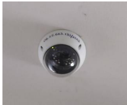
[S3] CCTV system.
