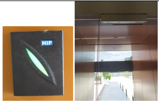
[S1]-Intruder alarm of Siri Varapunya building.
