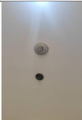
[S2] Fire-fighting system.
